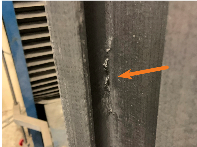
Figure 6: Two-foot span shear failure
