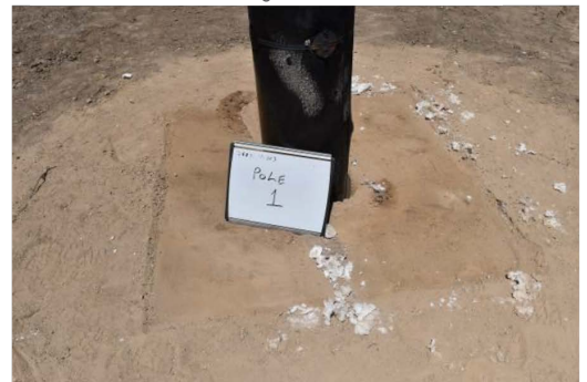
Post-Fire Exposure, Shroud Removed, Pole at Groundline
