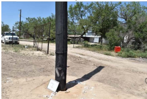
Post-Fire Exposure, Shroud Removed
