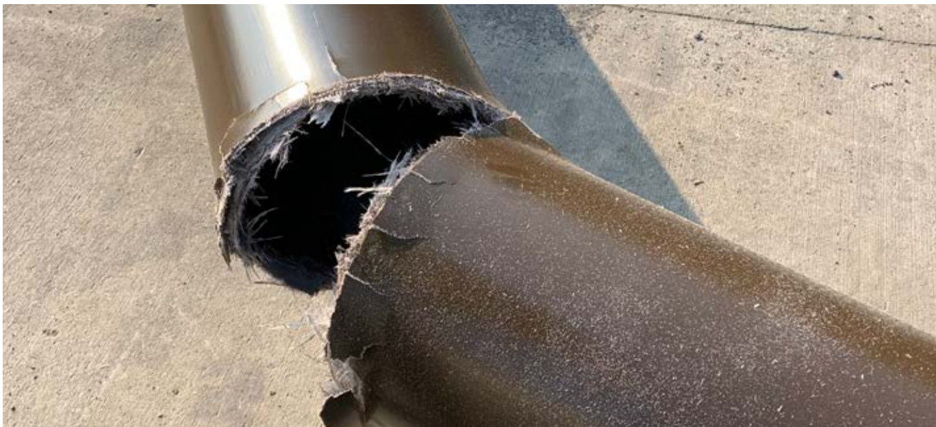
Photo of pole sheared by high velocity impact
