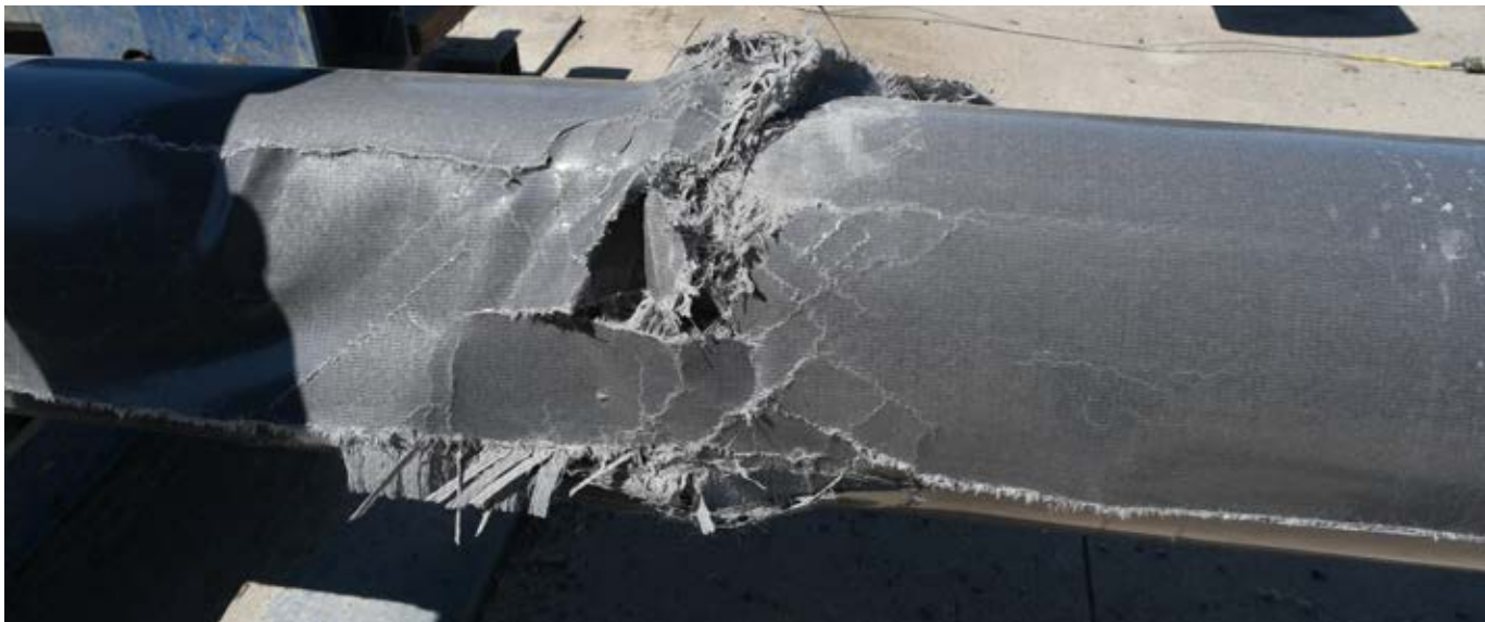
Photo of ruptured pole due to severe bending stress
