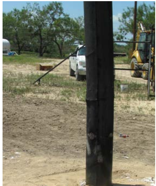
Photo of buckled pole, while its structural integrity appears to be intact, the pole should be replaced
